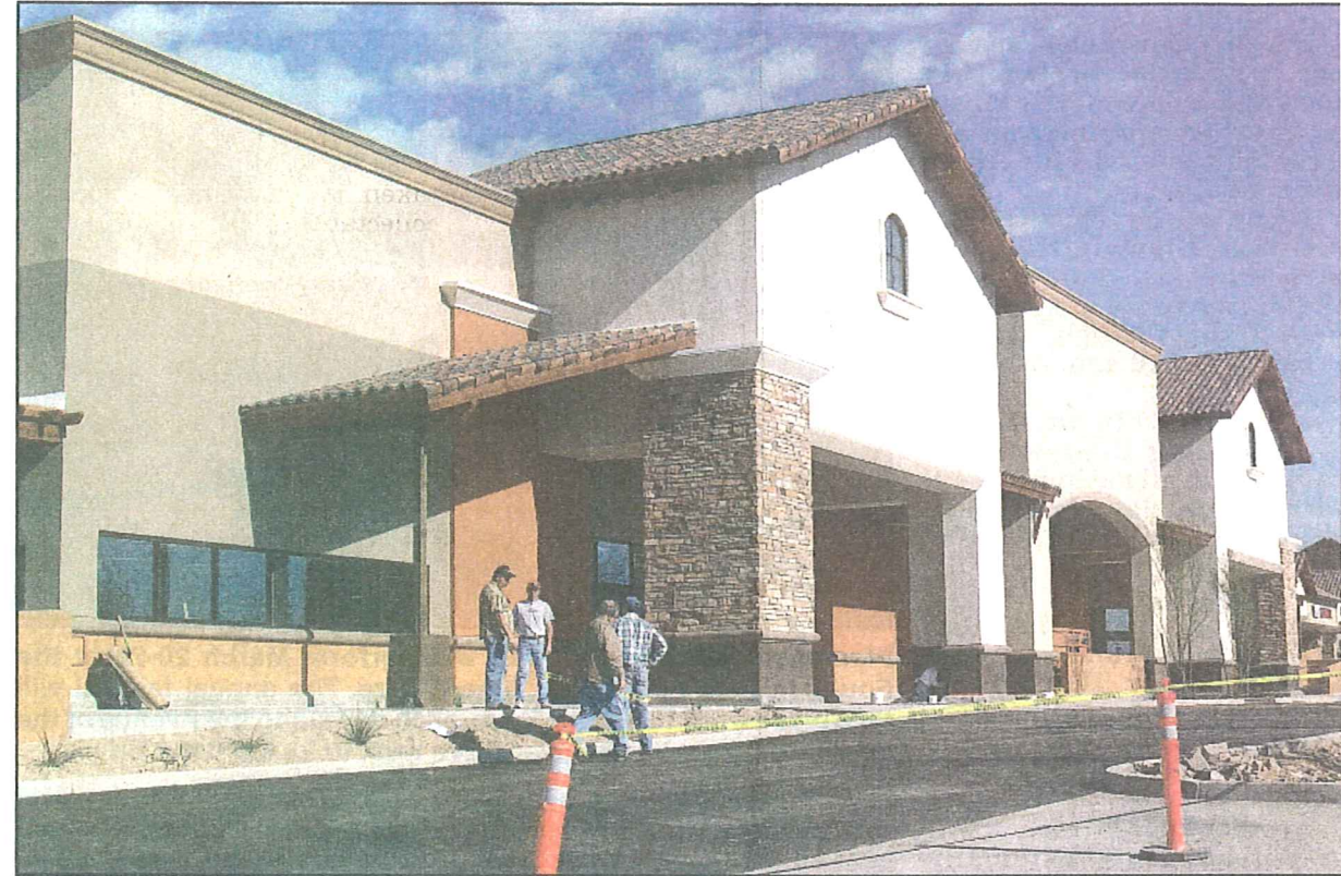
Crews make final improvements to the rebuilt, larger Bashas' supermarket at Fountain Hills Plaza, corner of Palisades Blvd. and La Montana Drive. The public is invited to preview the grocery store at 4 p.m., Tuesday, March 31.
